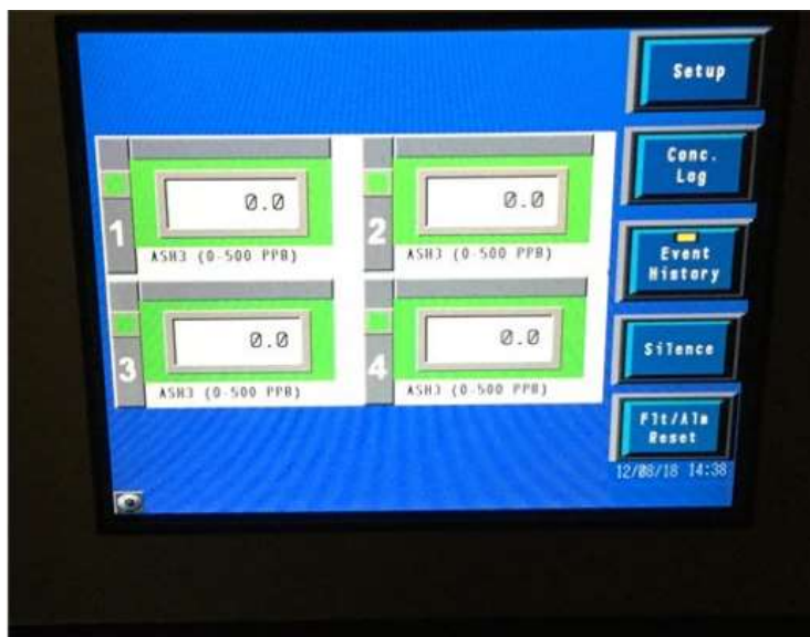
Figure 3: Gas sensors outside the lab door
